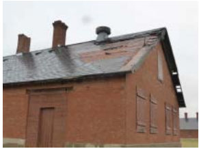
Fort Assiniboine wind storm damage; Hill County
